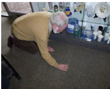
John having trouble with the cracks.
